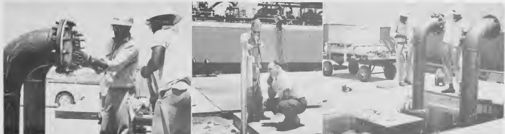
THE TWO men who connected the lines to the ammonia carrier were Calvin Schmidt and Adrian Wever. Pumping ammonia aboard the Esso Centro America actually began at about 5:30 p.m., Aug. 3. Moments after the pumping had been started, the pipes, above, turned white with frost caused by the extremely low temperatures which keep ammonia in a liquid state. In sixteen hours, 4000 tons of Aruba ammonia were loaded aboard the carrier.
